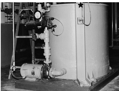
Reverse osmosis, Ósmosis invertida
