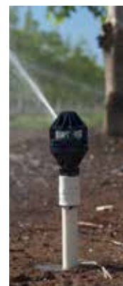
One of the most common methods of mounting an R2000 is on a PVC riser connected to an underground lateral line.
